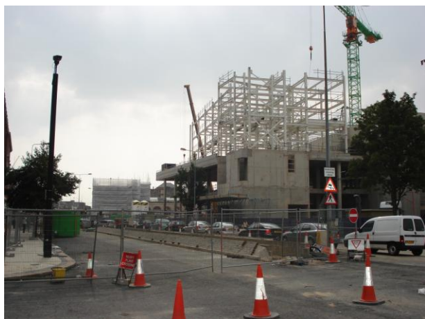
Ferensway: Paragon House (middle background) is encased in plastic sheeting ready for demolition, while the new hotel (foreground) takes shape and the central reservation walls are under construction. (Photo JD Scotney, September 2006)
