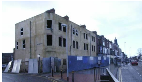
Anlaby Road – half-finished renovation of shops opposite West Park. (Photo: J.D. Scotney)
