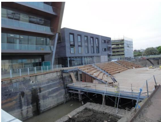
C4DI - second block unveiled and decking in Central Dry Dock (Photo: JDS)
