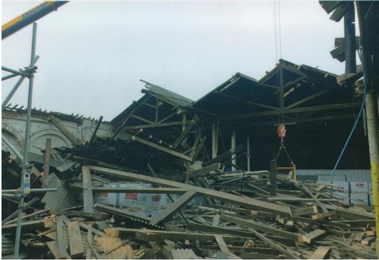
Another view of the storm damage (Photo by PBS Ltd)
